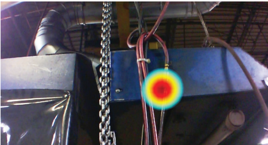
Image taken with the ii900 Industrial Acoustic Imager of an air leak in an industrial environment.
